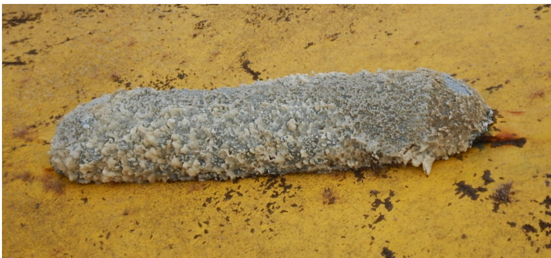
Figure 19 - Turbine Anode (before cleaning)
