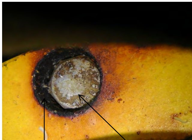
Carbon steel part corroded
