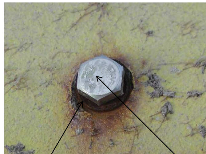
Carbon steel washer corroded
