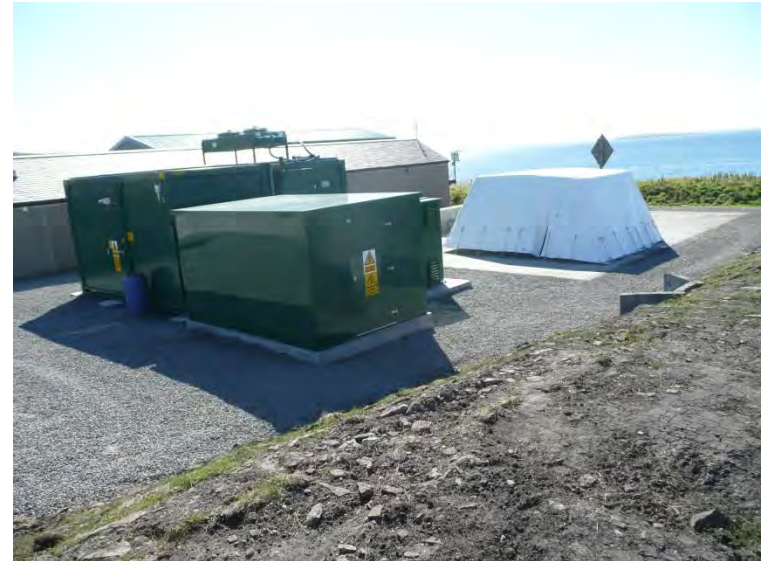
Transformer box at EMEC substation
