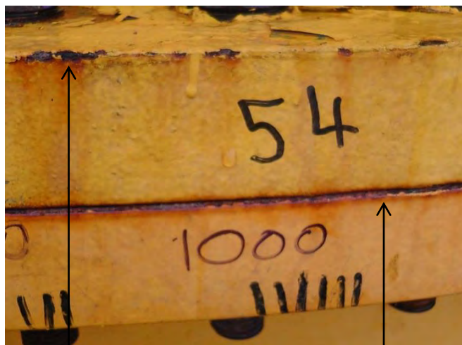
Paints cracks and corrosion
