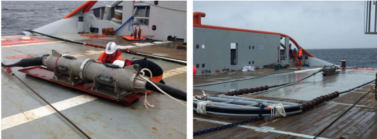
Figure 8. Connection and cable laying phases of the D10 turbine. Source: Sabella website
