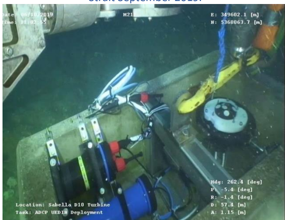
RealTide seabed sensor being left on seabed. The ROV is in the process of detaching the crane hook.
