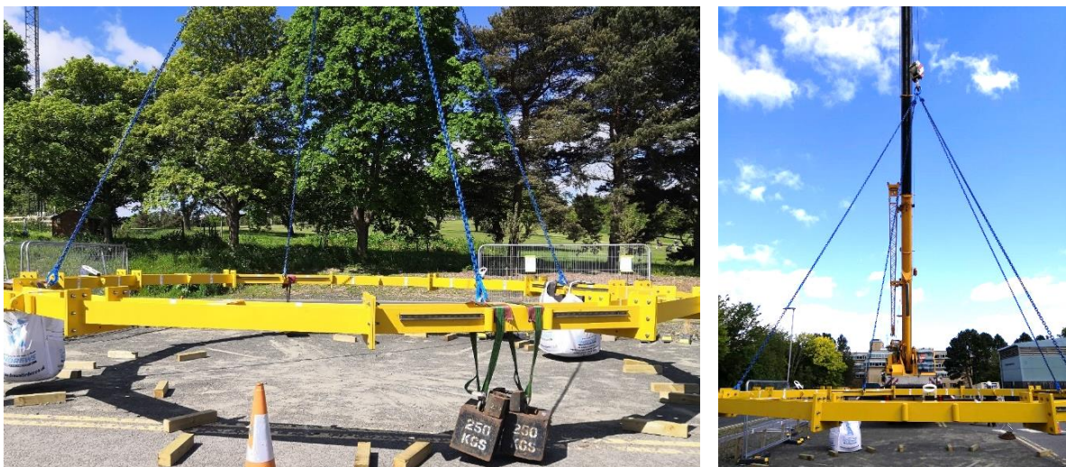
Figure 3-23. Lift testing of the C-ADP frame via the designed four-point lifting method, prior to dismantling and shipping to EMEC for re-assembly and instrument fit-out.
